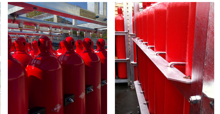
Earthquake Resistant Gas Cylinder Rack
